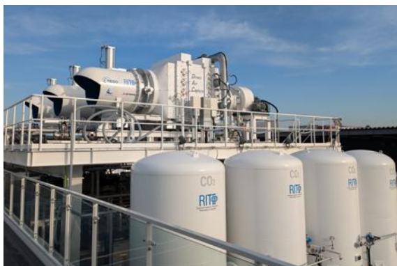
Fig. 4. CO 2 store tanks
