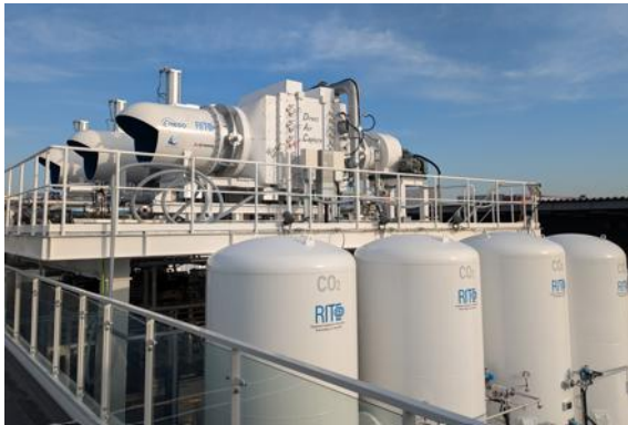
Fig. 4. CO 2 store tanks
