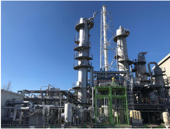
Fig. 1 Equipment of energy-saving CO 2 absorption process ESCAP® at Niihama Nishi power station, Sumitomo Joint Electric Power Co., Ltd.
